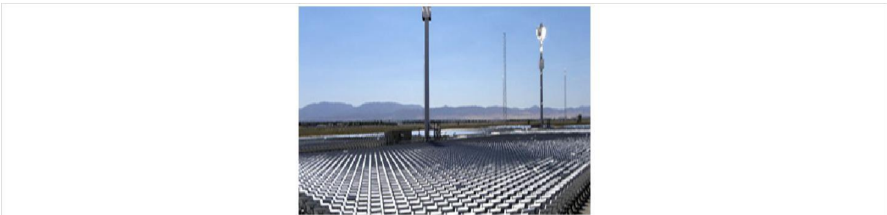
Solar power tower
